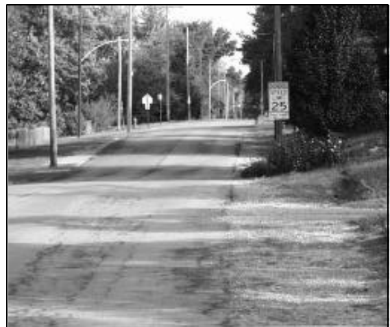
Curbs and sidewalks would enhance drainage, beautify streets and make walking easier and safer.
