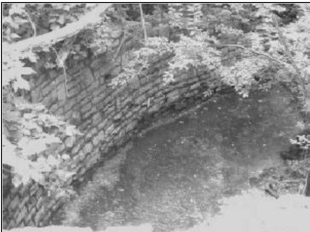
Open storm drain on 84 th and Main
